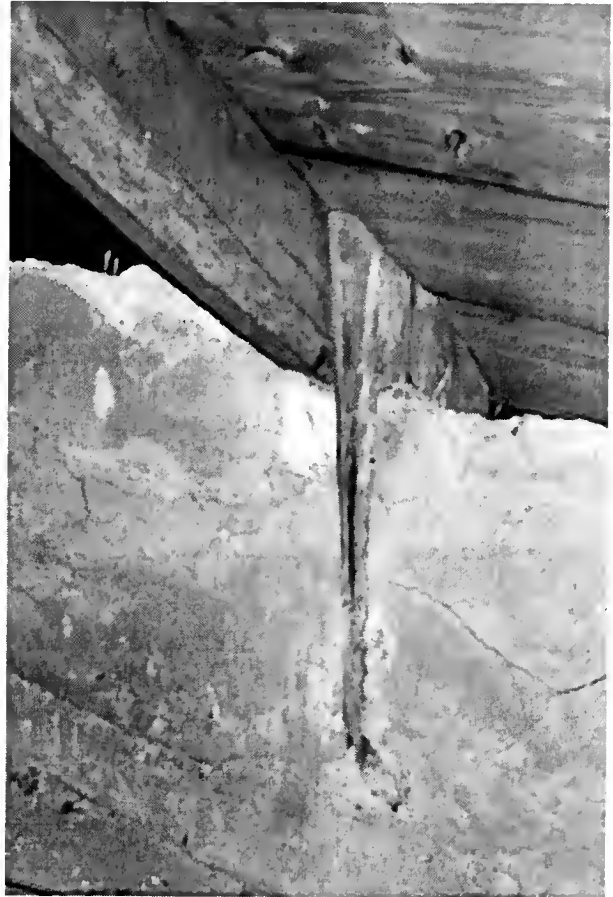
Figure 33 Remnant of Partition Wall in Attic of the Center Section of the Main House, 2002
